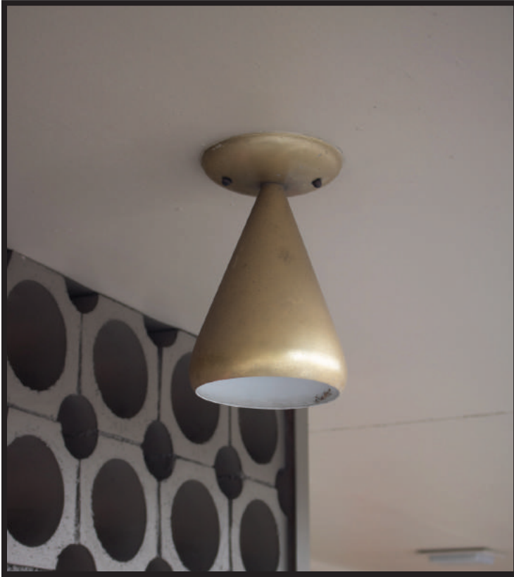
Figure 38. Typical Exterior Light Fixture
